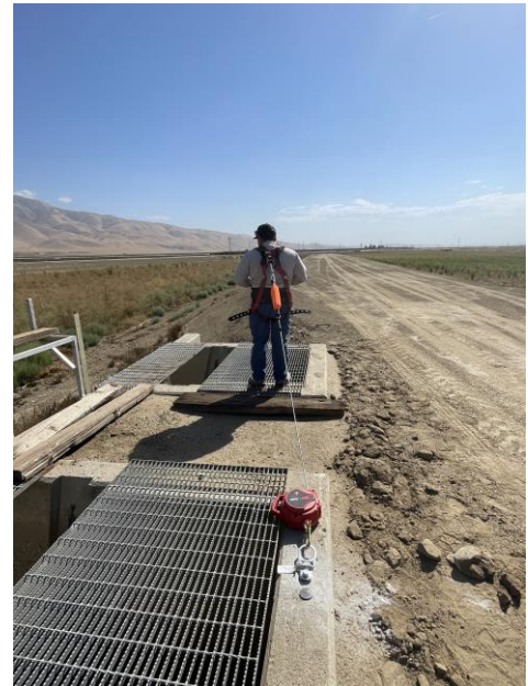
No Fall Equipment Installed on Interbasin Structures (Sycamore Spreading Row 1 Pond 1)
