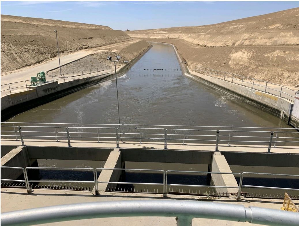
Pump and Power Testing at Forrest Frick Pumping Plant Forebay
