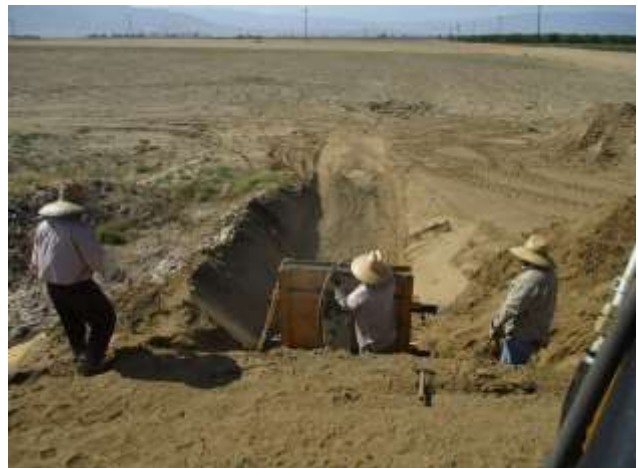
Concrete Pour for New Interbasin Structure Cutoff Wall (North Canal Spreading Works)
