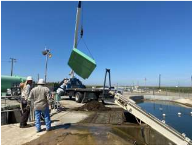
New Fabricated Moss Screen Trough (S73-P1)
