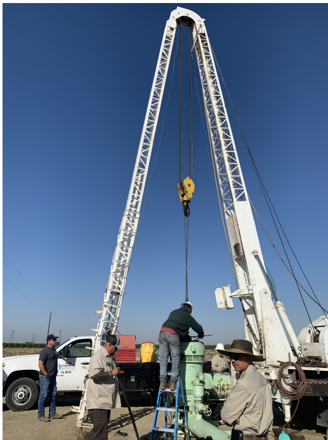
Startup at Sycamore Well #26
