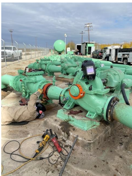
New Horizontal Pump Install
