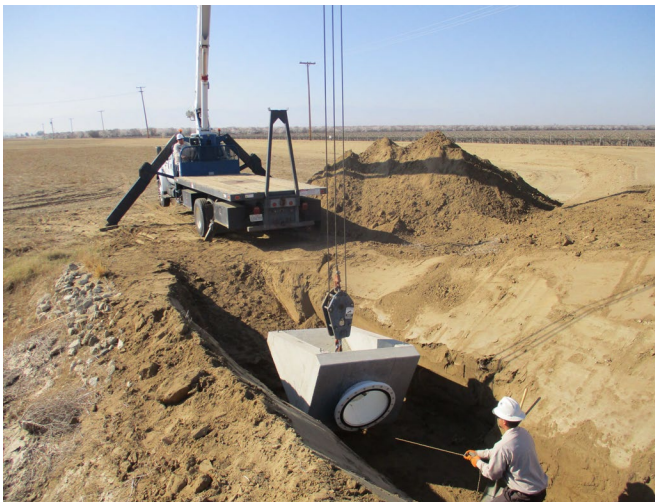
Interbasin Structure Installation to increase capacity into gravity ponds (NCSW)
