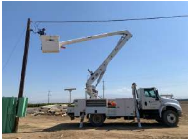
Replacing Burnt 3 Phase Connections for Construction Water (Sunset GW Recharge Facility Well)
