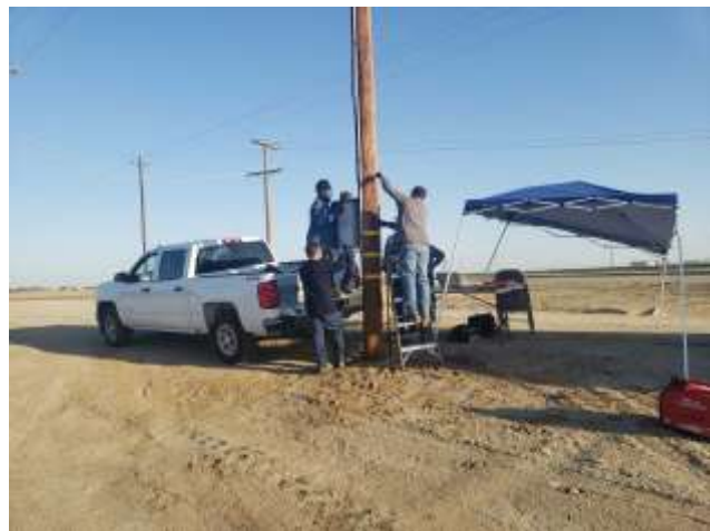
Recloser troubleshooting for Max Well Operation (North Canal Spreading Works)
