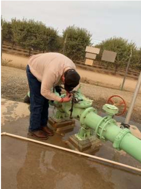
Clearing Out Filters on Bypass Valve (S73-P4)
