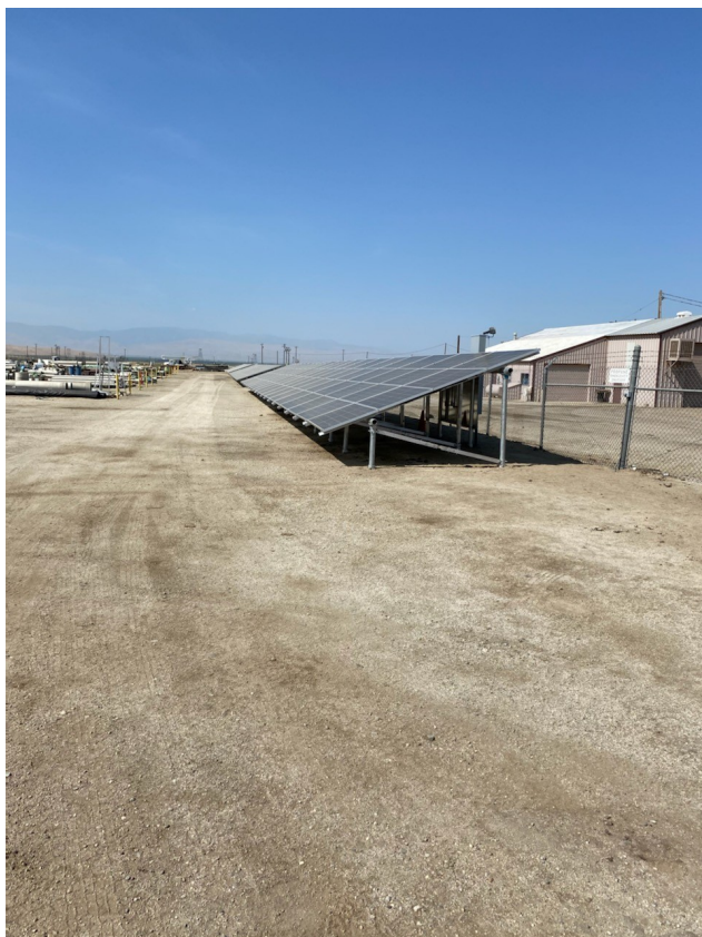
Solar Project Completed at District Headquarters
