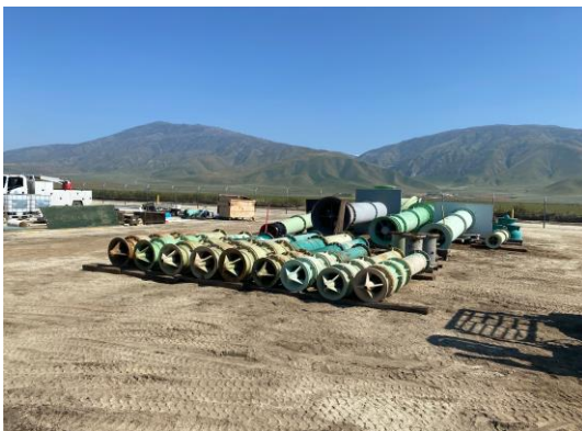
Organizing Pump Inventory (Headquarters)
